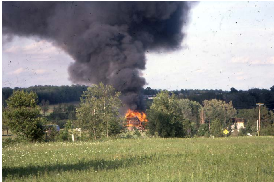
Razing of Buildings on the Gengler Farm in 1984 Photo by Loretta Kuse
